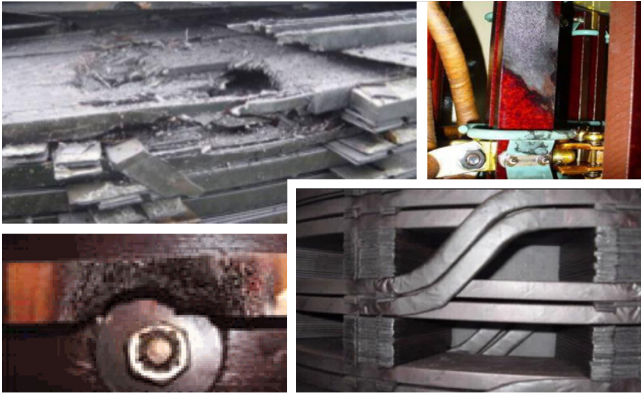
Figure 3. Fault examples (from the left to the bottom: D2, D1, T3 and T1), Cigre - JWG D1/A2.47 (2019)
